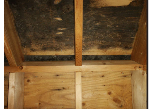
An attic view of the center ridge of a roof with algae on the north side of the roof.
